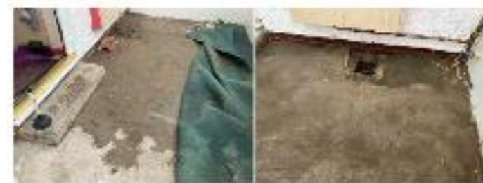
Crew have been shown to conservatory in the rear of the property that has been built. Customer has left external gully open which has flooded out. As per amendment, this is an external asset and therefore classified as external flooding only.
