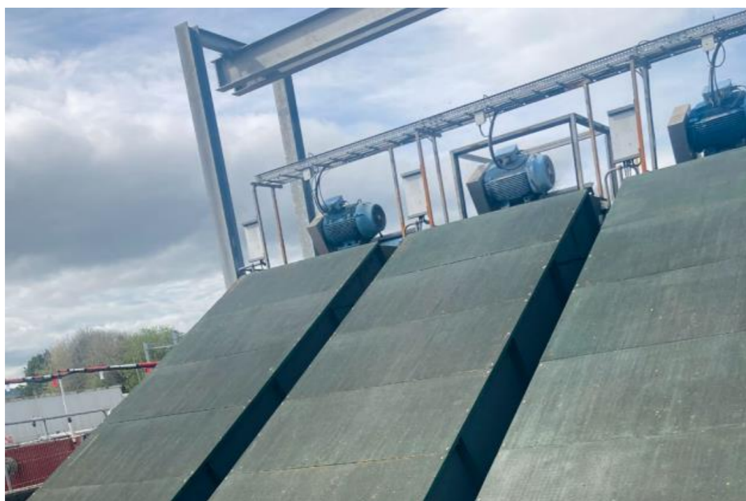
Barlaston screw pumps
