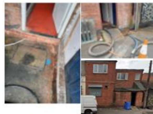
Crew shown to manhole extension at side of shop with EOS. Manhole is an external asset and has not been sealed when owner/resident has built over it. External flooding only.
