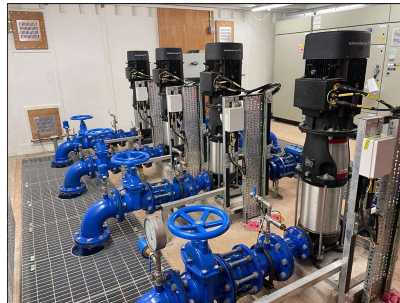
New LoS pumping station.
