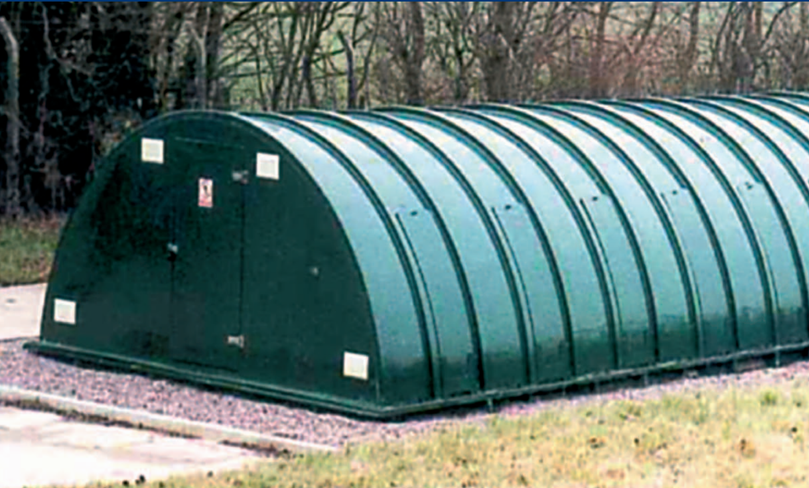
Rotating Biological Contactor (RBC)
