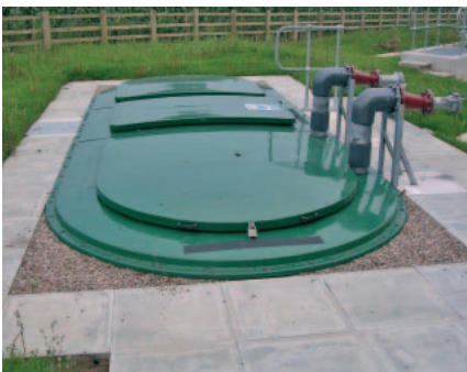
Submerged Aeration Filter (SAF)
