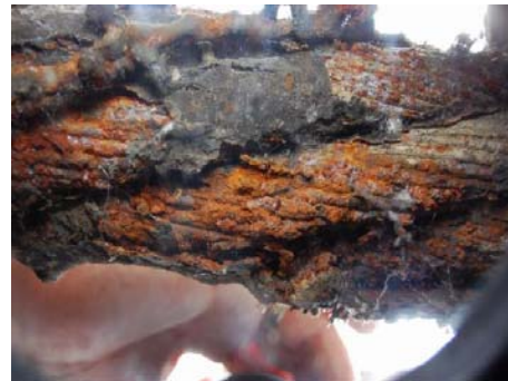
Corrosion to Catenary Cables Adjacent Anchorage Chamber Entry
