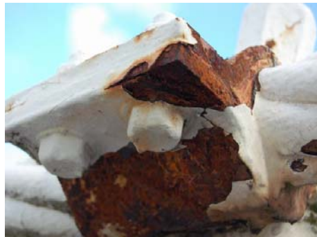
Corrosion to Cable Band Plates
