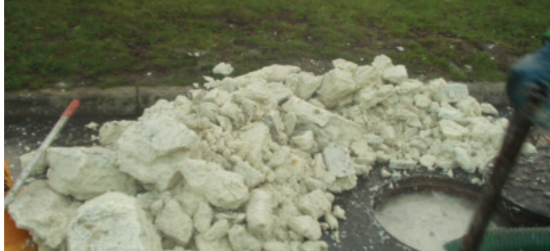
fat oils and grease removed from a Severn Trent Water sewer
